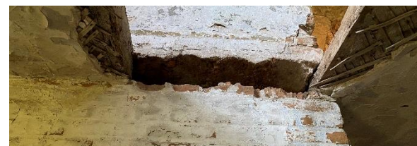
Figure 3 – First floor ceiling: 1 – finish floorboards, 4.5 cm thick; 2 – subfloor boards, 6.5 cm thick; 3 – joists, 30 cm wide, 22 cm high; 4–5 – lime plaster on lath
