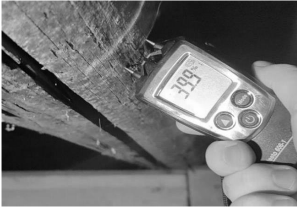
Figure 5 - The results of the moisture measurement of wooden rafters were performed using a Testo 606-1 moisture meter.
