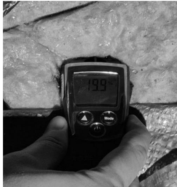
Figure 8 - Increased humidity of mineral wool at attic level
