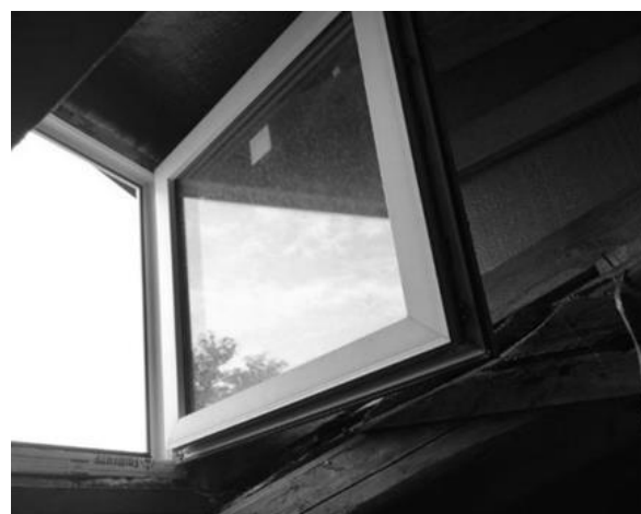
Figure 4 - Hermetic metal-plastic windows in attic openings, which negatively affect the ventilation of the attic space
