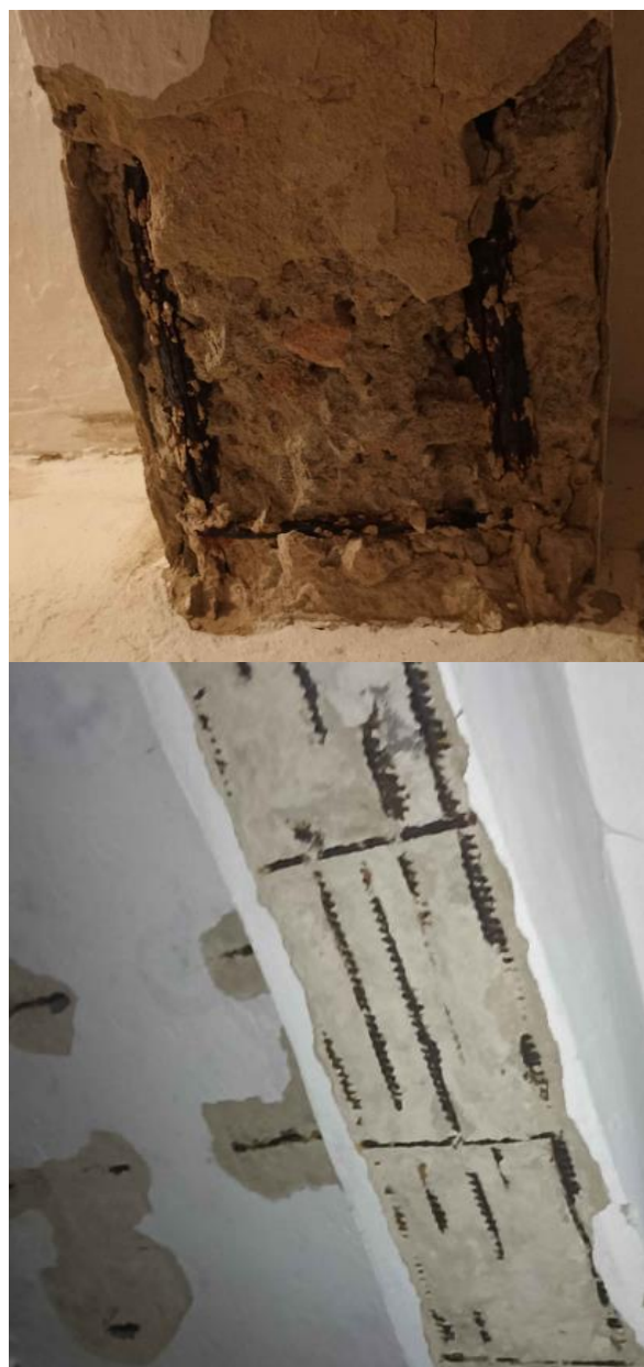
Figure 2 – Detachment of the protective layer of concrete in the reinforced concrete floor beams of the basement.
