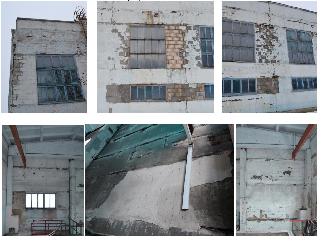
Figure 7 – Damage to wall panels
