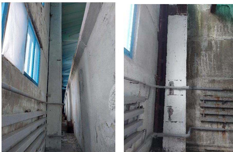
Figure 4 – Damage to reinforced concrete columns of the outer rows
