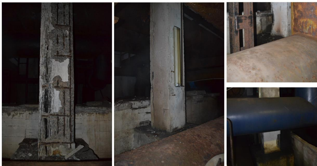
Figure 3 – Damage to reinforced concrete columns of the middle row
