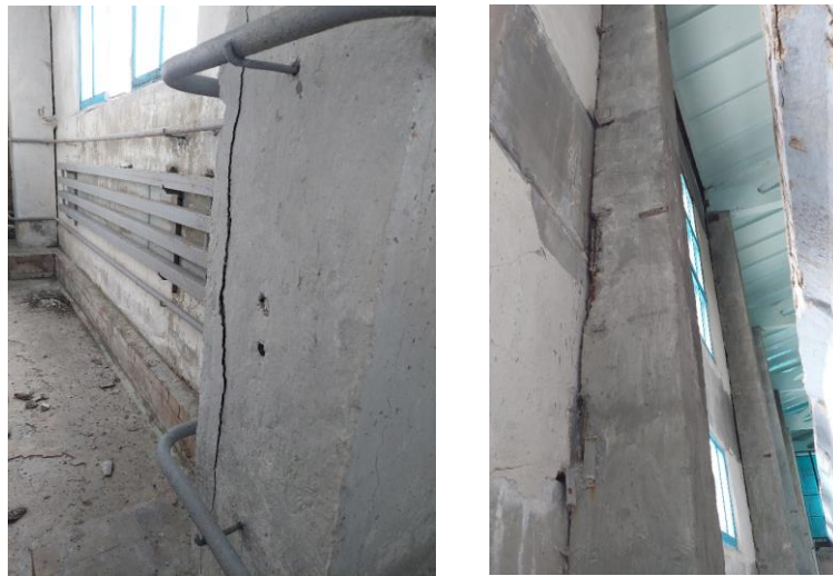
Figure 5 – Damage to reinforced concrete columns of the outer rows
